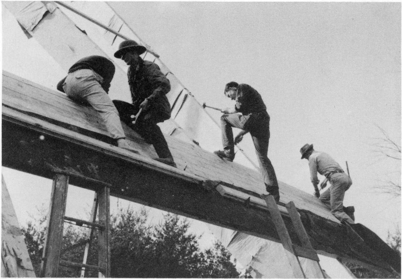
Students working on construction of new chapel—Completed in 1967, the chapel houses the Warren Wilson Presbyterian Church.
